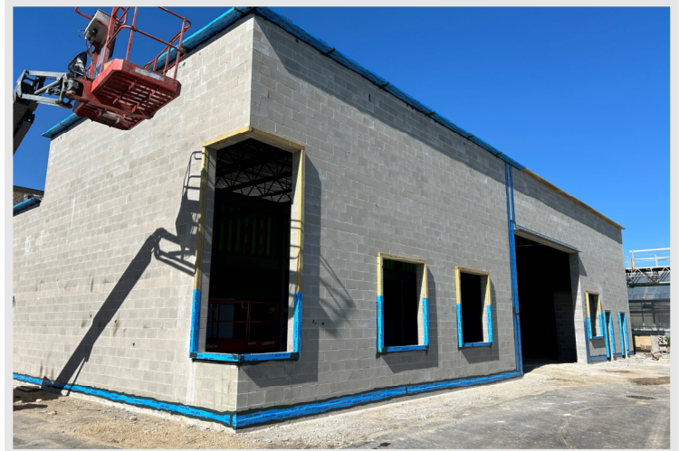
Air/vapor barrier detailing work continues at the Skills Lab Addition, spray application of the barrier will follow shortly behind.
